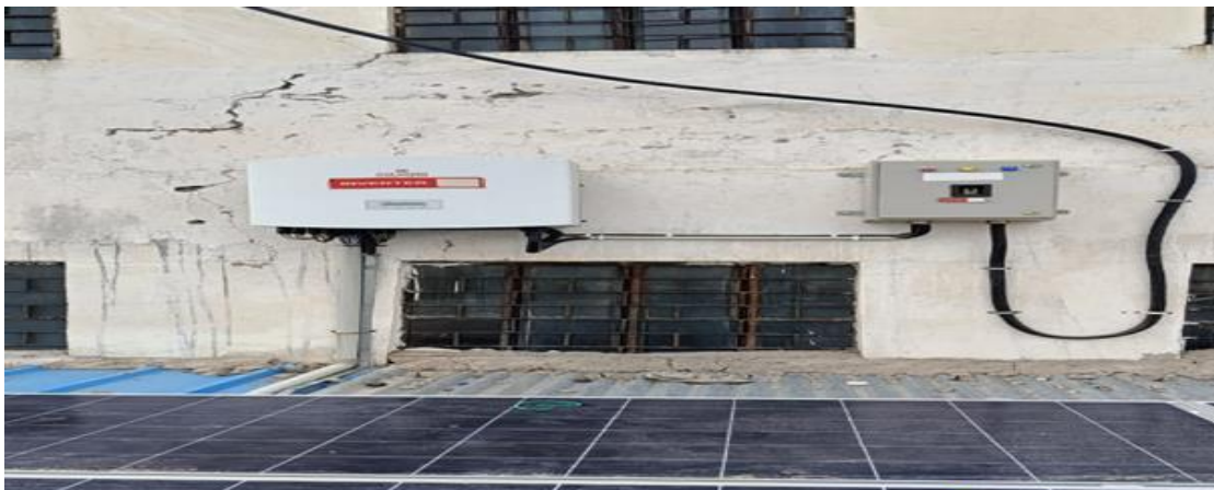
Solar Energy System in Campus
